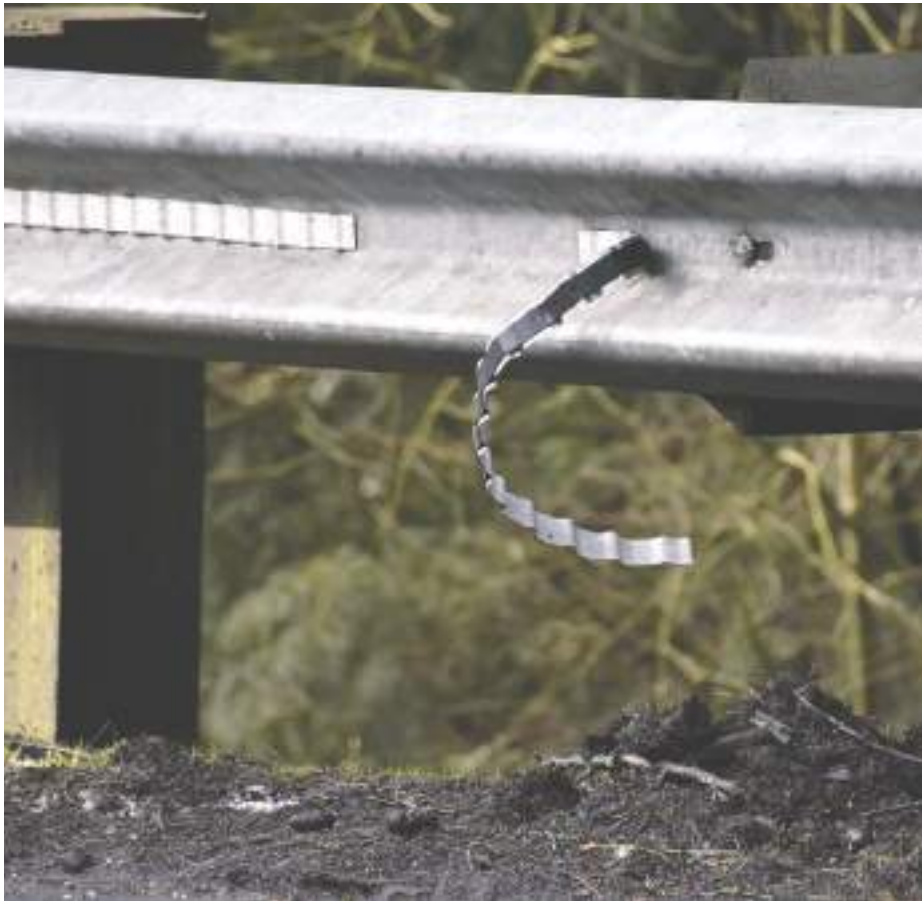
Reflective tape applied to guardrails on SR 302 in 2014-15 started peeling off during the cold spell in December 2016. According to sources at WSDOT, the steel might not have been well prepped before the tape was applied, the adhesive might have been bad or it might not be up to the freezing weather, but no one is sure why it's failing. Photo: Don Tjossem, KP News
