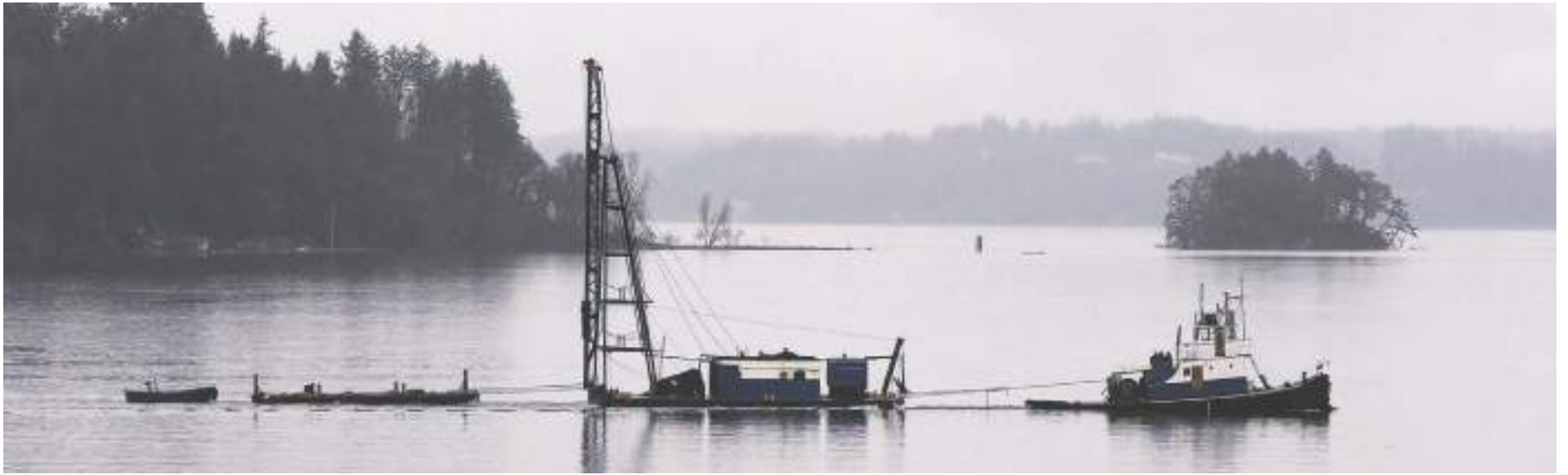
Its work finished for now, the work barge is towed out of Filucy Bay on an overcast February day. Photo: Richard Hildahl
