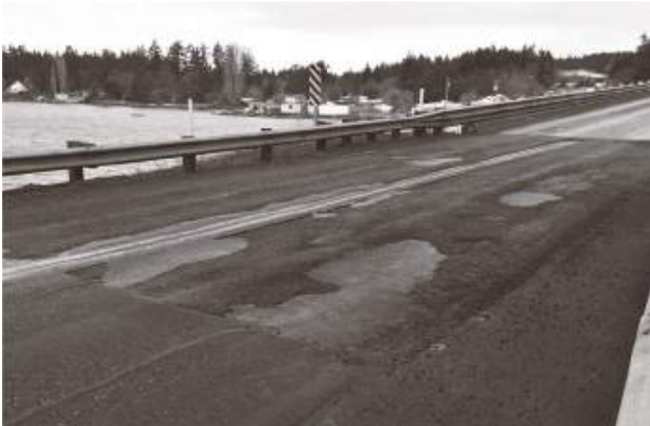
Recent repair work on the Purdy Bridge is coming apart. Photo: Don Tjossem, KP News
