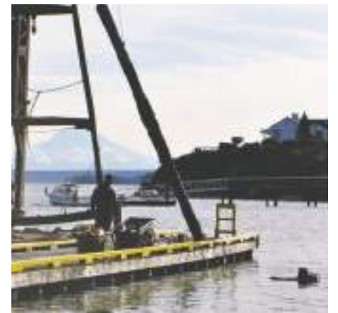
A work barge pulls an old piling from the Longbranch Marina dock. The diver in the water cut off the piling at the mud line using a compressed-air-driven chain saw. Photo: Lynn Carr
