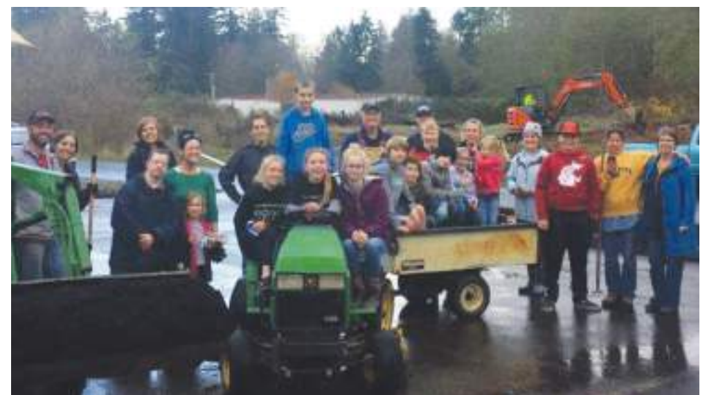
On Nov. 18, Dale Christensen from Christensen Construction and Ryan Barringer from Silver Bow Farm started clearing land for the future Mustard Seed Project senior housing site opposite the former Roadhouse restaurant in Key Center. The next day, Lynn Christensen led about 30 landscaping volunteers from Harbor Christian Center and a few from TMSP. The Christensens secured a large dump truck load of donated mulch from Peninsula Topsoil in Belfair. The Mustard Seed Project is very grateful for everyone's efforts. Photo: Robyn Readwin, TMSP
