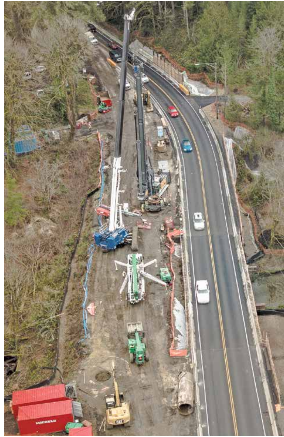
With the temporary two-lane bypass complete to relieve traffic impacts on SR-302, the next phase of the $16 million bridge construction project began to replace three outdated culverts to allow fish passage. Four drilled shafts approximately six feet in diameter and 50 feet deep into the earth were completed Feb. 12. They will provide a solid foundation for the new bridge to be built over Minter Creek Photo: Jim Bellamy
