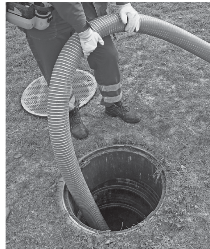
Pumping out a holding tank is a costly option. Photo: AdobeStock
