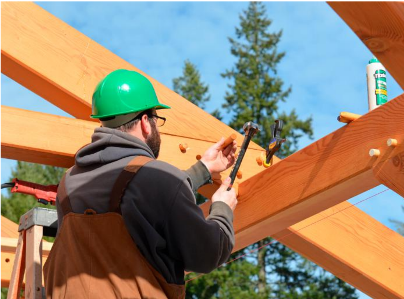
Eddie Vannausdle adds anchor pegs to joints in new open-span timber structure. Photo: Lisa Bryan, KP News
