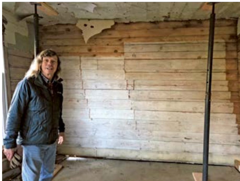
Bart Wolfe describes how joinery in the library wall that stood straight for a century was forced out of alignment by the crash. Ted Olinger, KP News
